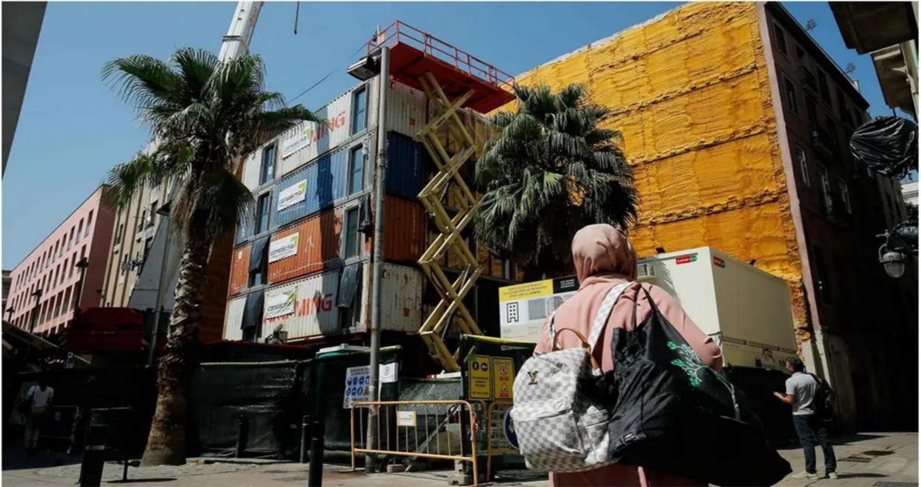
▲ People walk by the construction site of the first building built with shipping containers in Barcelona. Photograph: Pau Barrena/AFP/Getty Images
